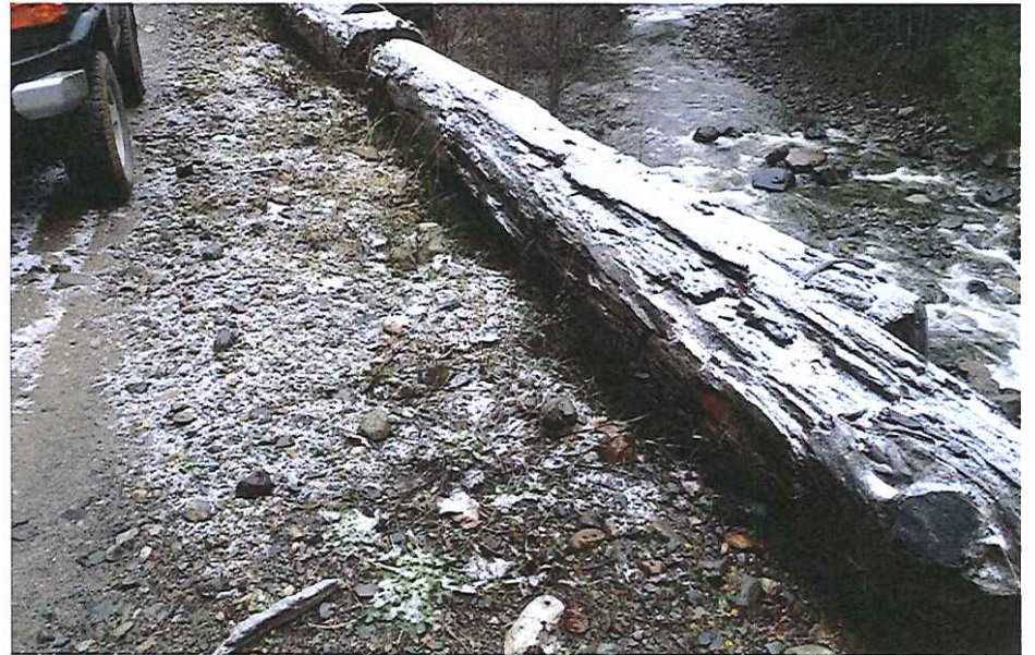
CK2236 Deck fill eroding
